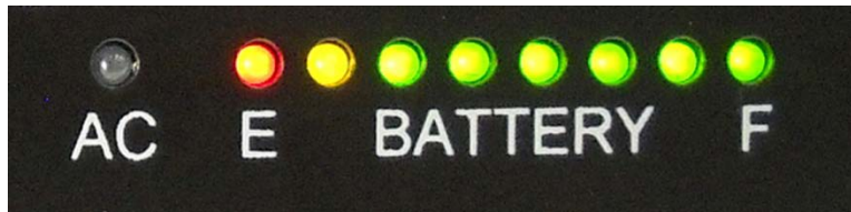
Battery “Fuel Gauge” indicating a fully charged battery
