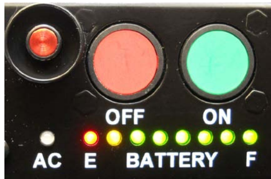
Battery “Fuel Gauge” indicating a fully charged battery
